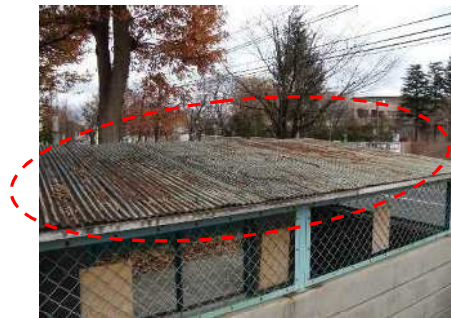
●ゴミ置場屋根の錆
