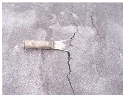
●防水層の破断*2
